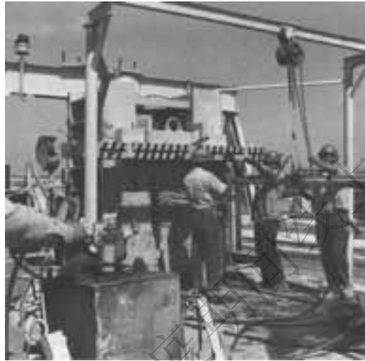
Fig. 2-5 Massive strand jacking abutment at the end of a long pretensioning bed (Courtesy of Concrete Technology Corporation).
