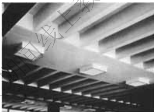
Fig. 1-2 One-way joist floor system, with closely spaced ribs supported by monolithic concrete beams; transverse ribs provide for lateral distribution of localized loads (Portland Cement Association).
