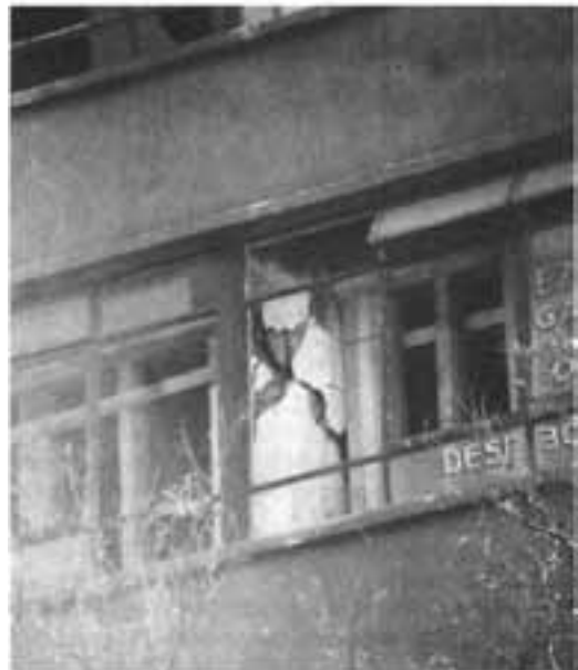
Fig. 4-6 Shear failure in a captive column without adequate transverse reinforcement.
