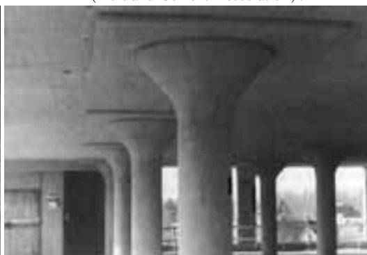
Fig. 1-4 Flat slab floor, without beams but with slab thickness increased at the columns and with flared column tops to provide for local stress concentration of forces.
