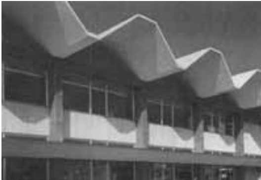
Fig. 1-5 Folded plate roof of 125 ft span, in addition to carrying ordinary roof loads, carries the second floor as well from a system of cable hangers; the ground floor is kept free of columns.
