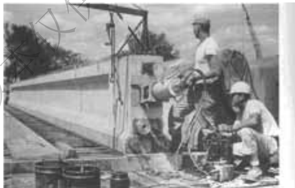
Fig. 2-6 Post-tensioning a bridge girder: use a portable jack to stress multistrand tendons (Courtesy of Concrete Technology Corporation).
