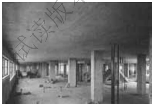
Fig. 1-3 Flat plate floor slab, carried directly by columns without beams or girders (Portland Cement Association).
